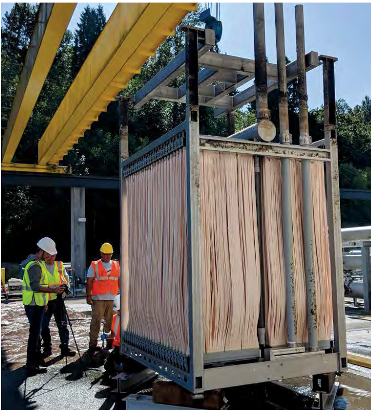
A 2019 upgrade of the “membrane bioreactor” (MBR) at the Brightwater wastewater treatment plant is saving the facility over 2,000,000 kilowatt-hours of electricity each year. The MBR process is a crucial step in creating the high-quality effluent (treated wastewater) produced at Brightwater.
