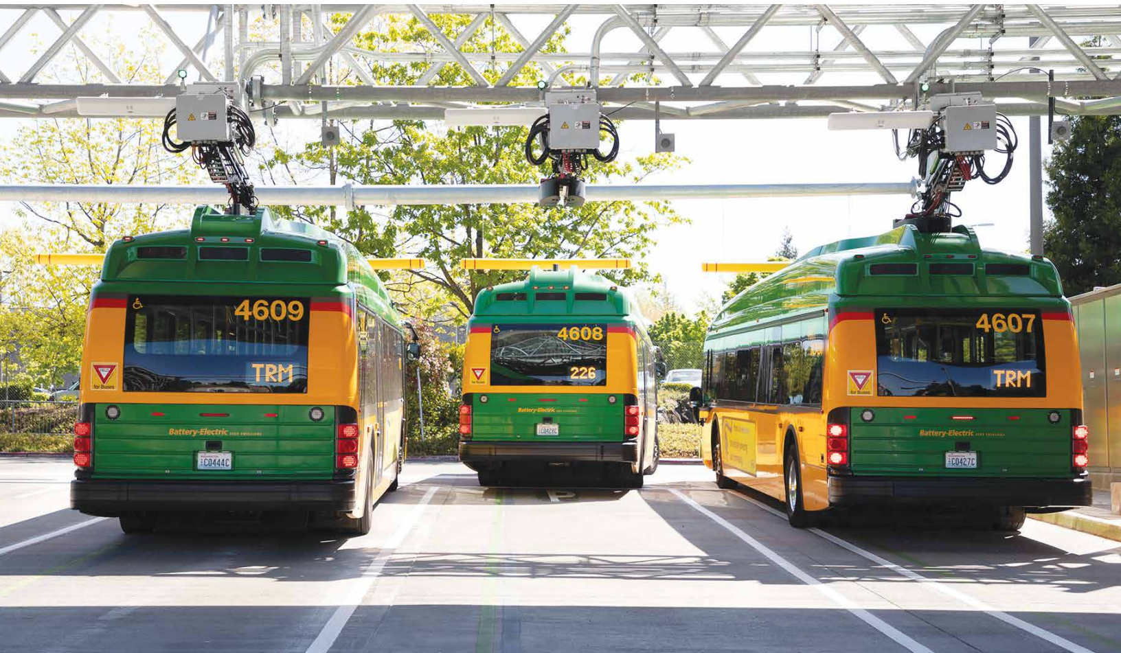
Battery electric buses charging at Eastgate Park-and-Ride.
