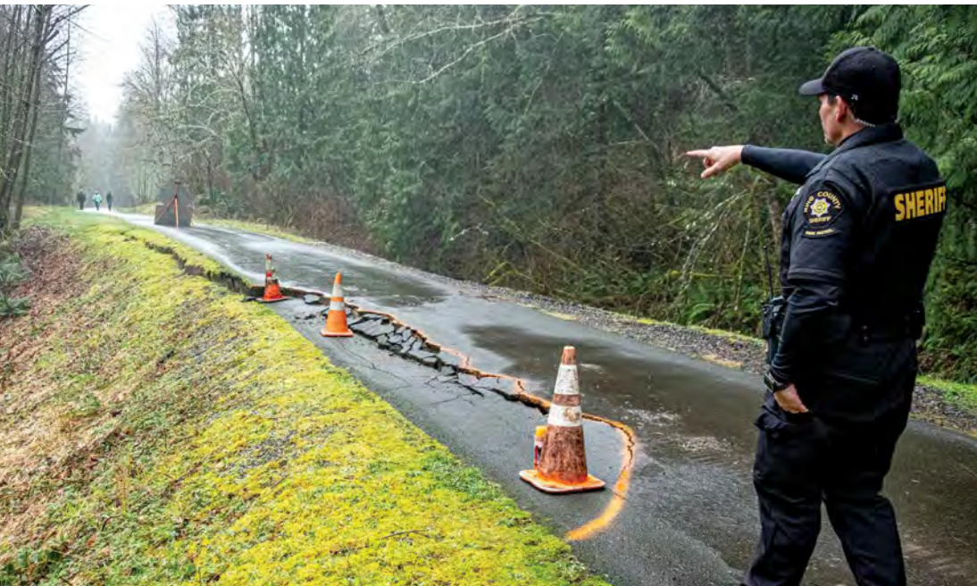
Landslide along the Preston Lake Alice Trail, January 2020
