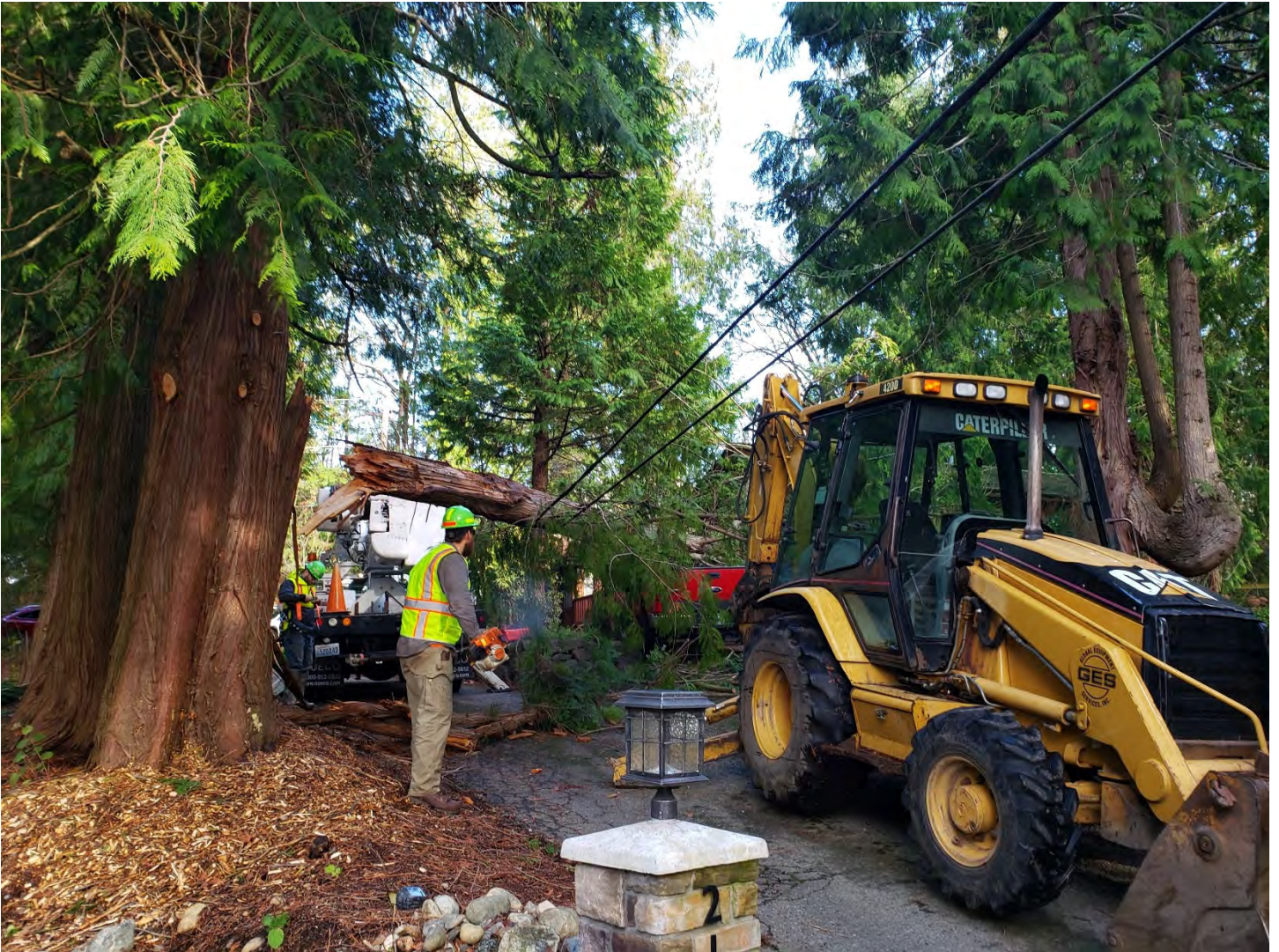
Public Works Maintenance Workers responding to a fallen tree, Maple Valley
